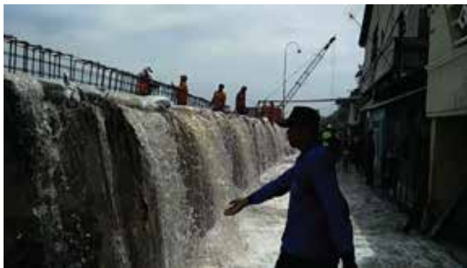
Figure 29. Construction of embankment along the coast to prevent tidal flooding caused by land subsidence in Jakarta
