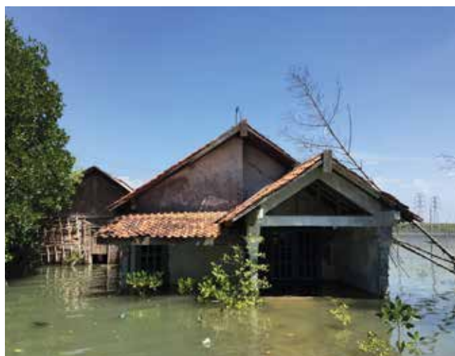
Figure 1. Deteriorated buildings in Semarang Utara and sinking houses in Sriwulan, Sayung, Demak due to land subsidence in the north coast of Central Java
