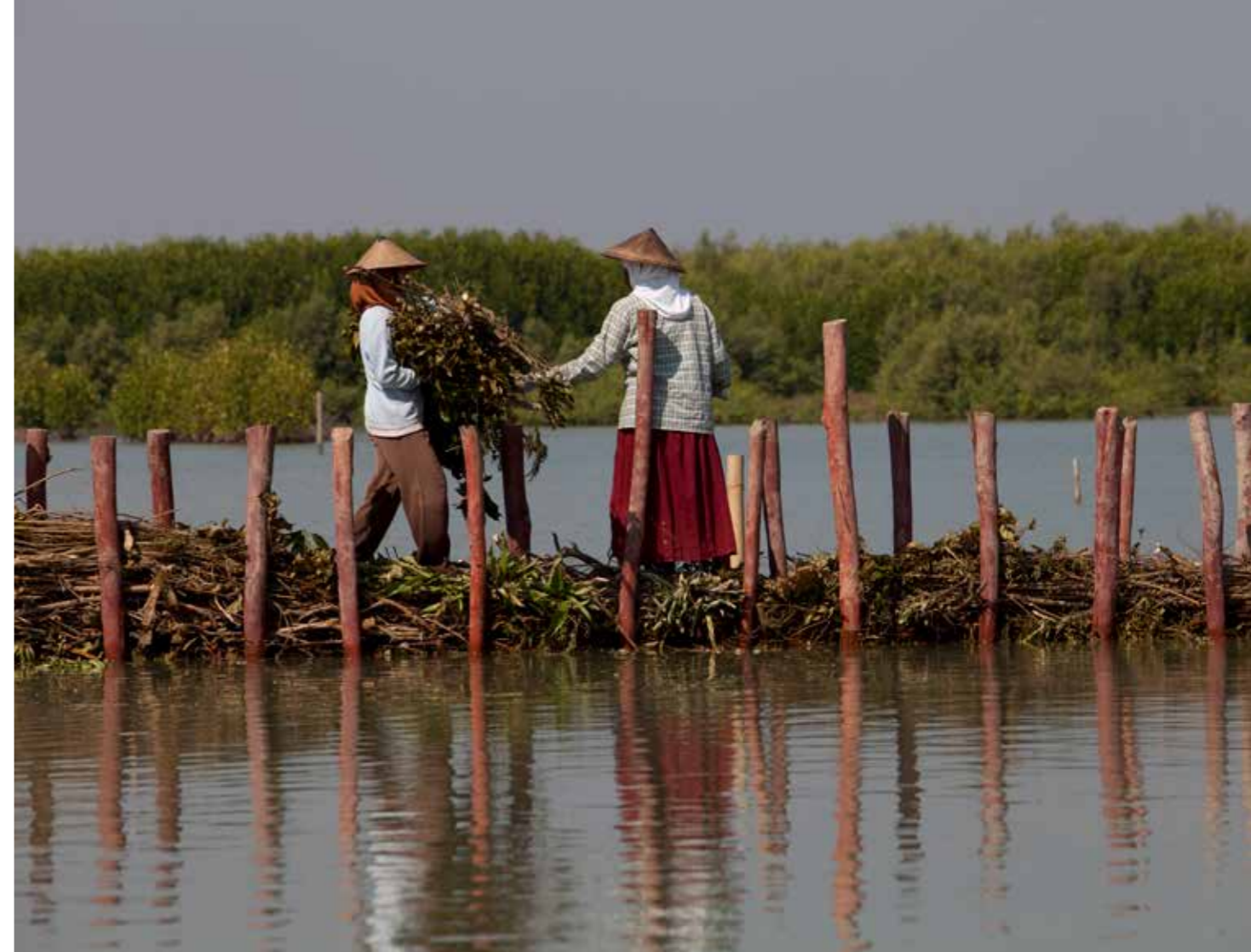
The local community helped build permeable structures in Demak, recompensed with financial support and training for new local economic activities.
