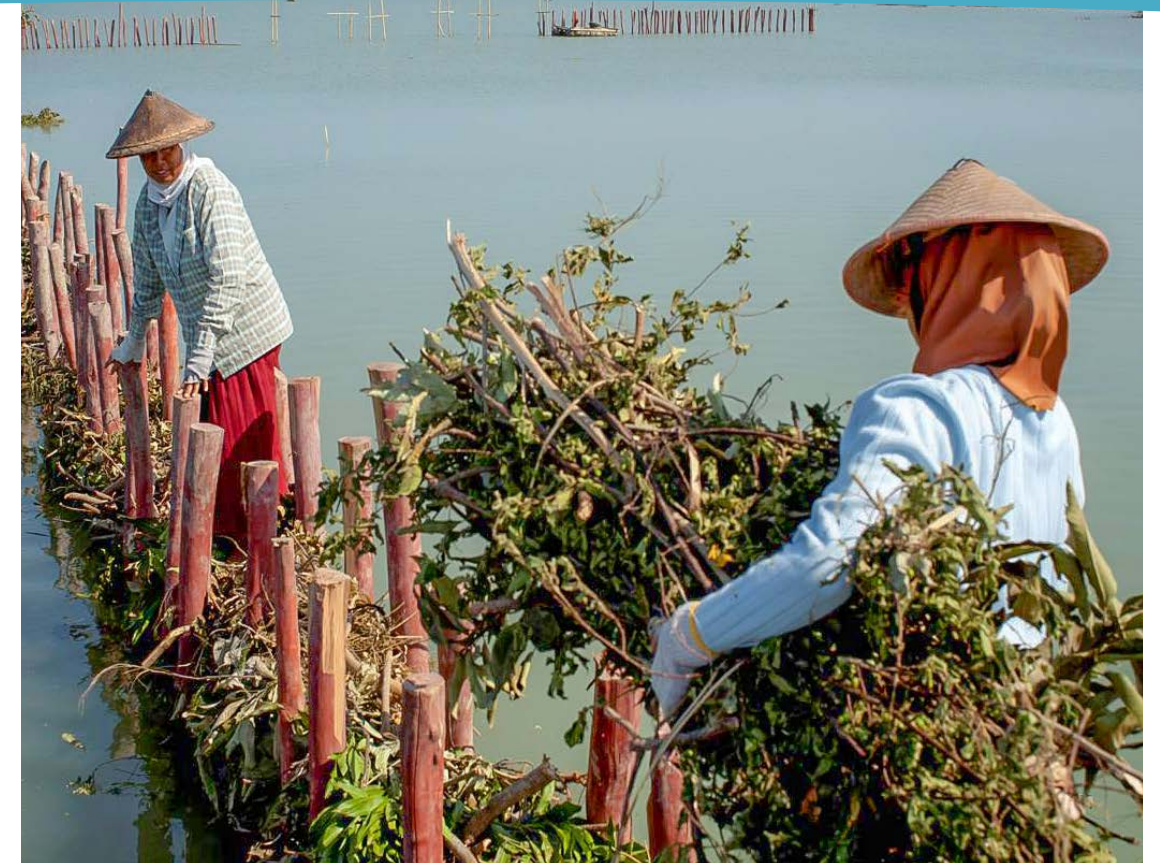
Figure 2. Construction of permeable structures by local women in Timbulloko (Demak, Indonesia) © Nanang Sujana
