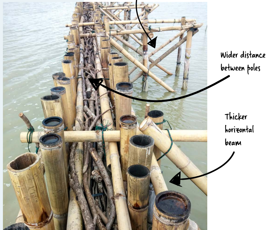
Figure 12. Alternative design that has more width between poles, support structure at the back, thicker horizontal beam © Tom Wilms, Witteveen+Bos
