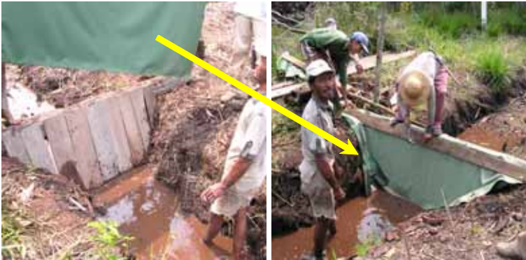
Illustration 50. Attaching the Plastic or Tarpaulin to the Wall of the Block (Photograph: Alue Dohong, 2003)
