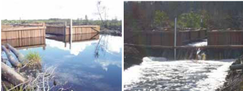
Illustration 72. Construction of Block in ex-PT SSI Canal after Completion (Documentation: WWF-Indonesia/ Drasopolino, 2004)
