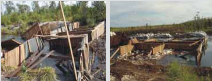
Blocks that were built on the upstream (left) and downstream (right) of the ex-canal of PT SSI were damaged by strong currents in January 2005 (Documentation WWF-I, Sebangau 2005).
