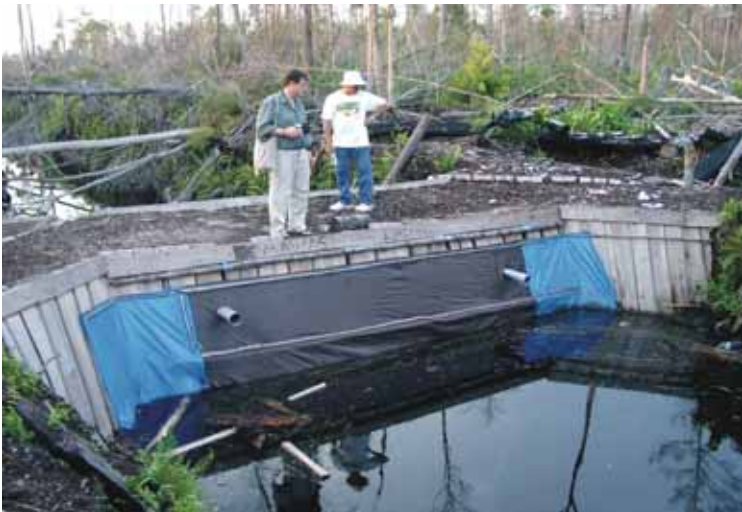
Illustration 11. Composite dam built by Yayasan MAWAS - BOS in one of eks-Mega Rice Project's canal, Kalimantan Tengah
