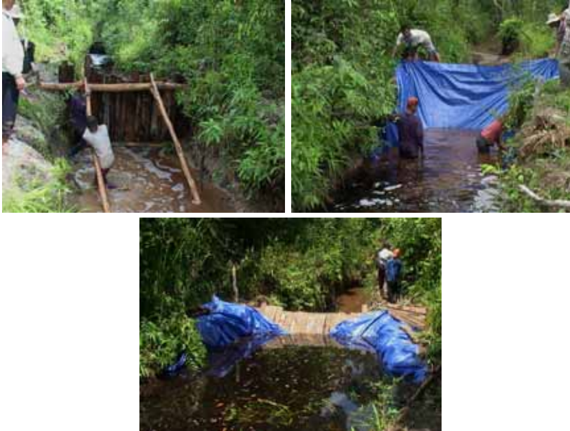
Illustration 76. Stages of building the temporary blocks by CCFPI in the ditch owned by Nasir (coordinates: S 01°57'34.0", E 103°59'08.7"). This block was later damaged by unknown illegal loggers. (Photograph: Suryadiputra, 2004)
