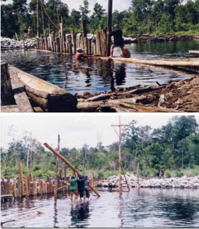
Illustration 30. Workers inserting the wood poles (top) and lifting the joining belangiran pole (Photograph: Suryadiputra 2004).
