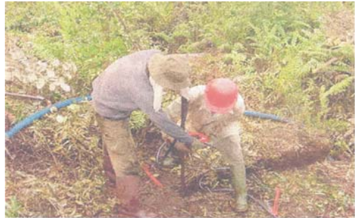
Sinking wells along the length of the fire break as sources of water for fire suppression (TSA CIMTROP UNPAR)
